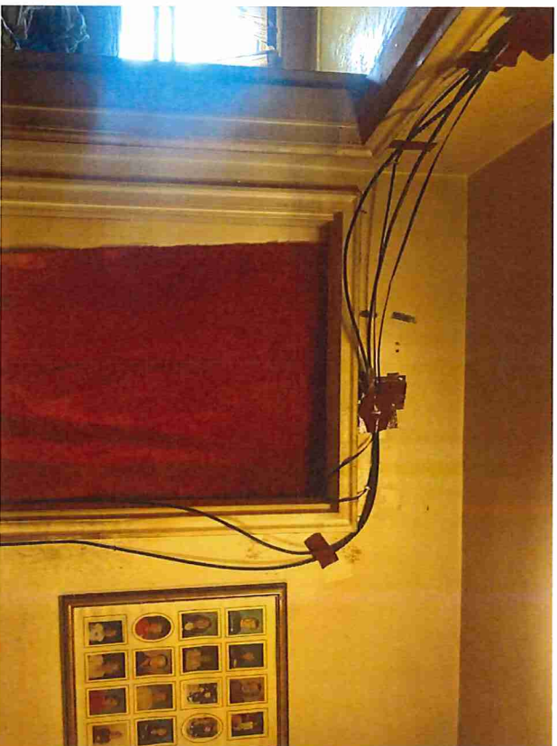
Inside cable wiring
